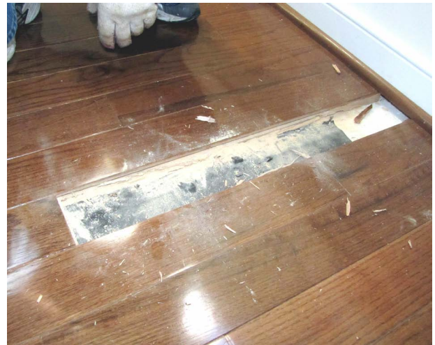
Replacing a section of powderpost beetle-infested and damaged wood is a nonchemical control option (Pinto)
